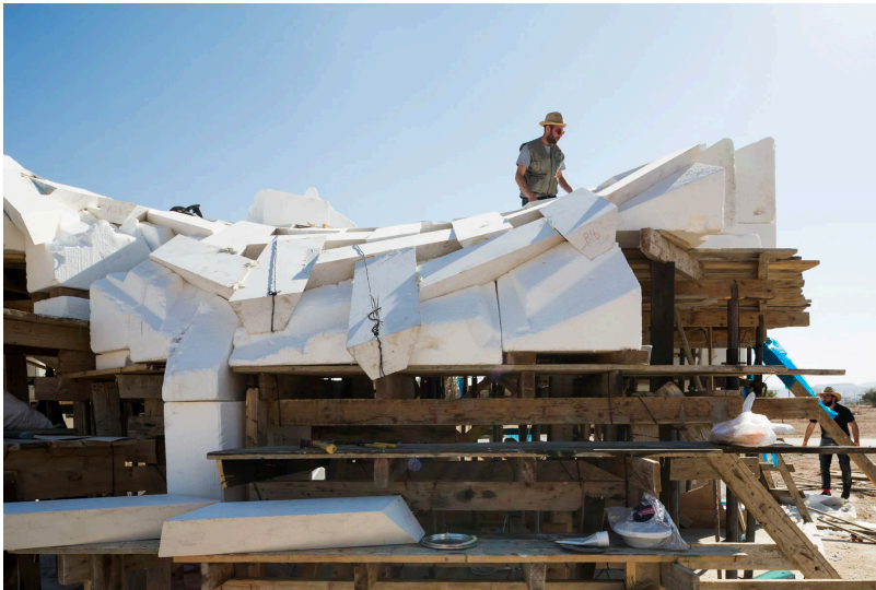
Construction on the vault of the el-Atlal artist residency project. Courtesy of AAU Anastas.
